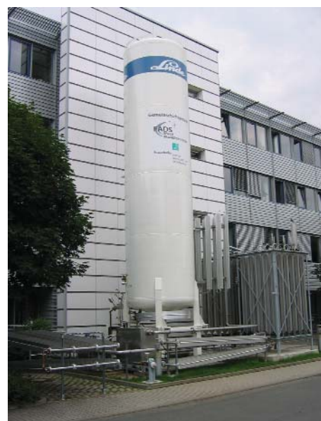
Nitrogen supply tank with delivery, mixing, and control system
